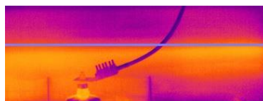
Figure 9: Oil level line of conservator
