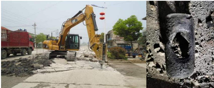
Fig. 1.1 Scene photo of gas pipeline failure
